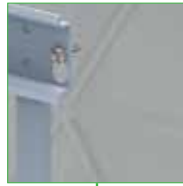
large space for cables
